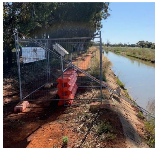
Figure 5: Temporary SL1500-3G Mounting Frame.
